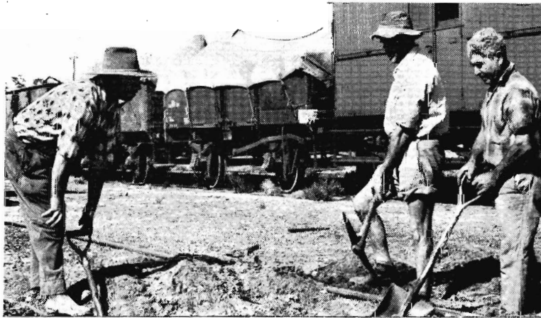
Members of gang No. 28 are at work in the Irymple yard. From left: Repairer D. C. Maizey, Actg. Ganger G. E. Perry, and Repairer A. Di Masi. The gang won first prize in its section of the 1968 track competitions.
