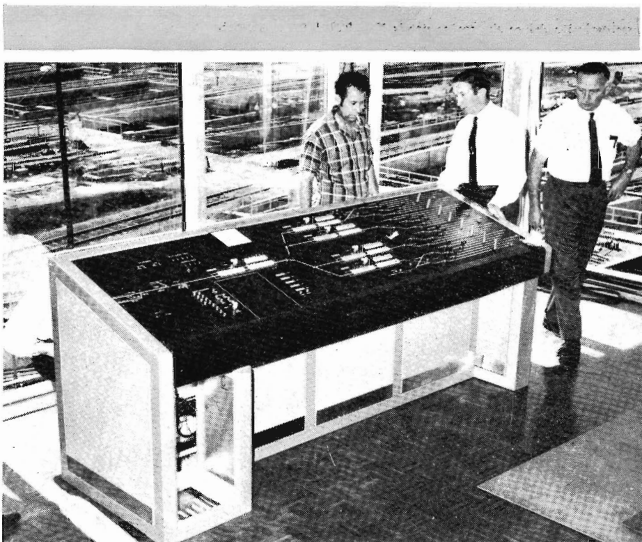
The installation last month of this retarder control console in the Melbourne Yard 70-ft. high West Tower brought the introduction of hump shunting another step closer. The console operator will monitor five retarders and the approaches to the hump, and set-up automatic switching to 32 sorting sidings.
